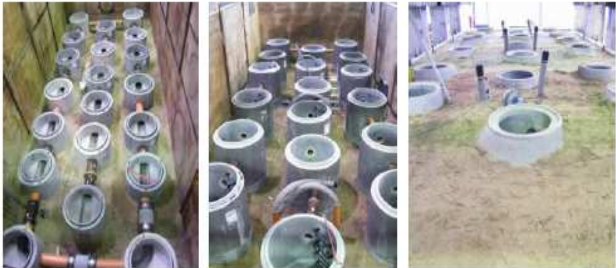
Photo 3: Installation of shafts in the test series as: Lower pipe layer DN 300 (left); medium pipe layer DN 150 (center); completed installation (right)
