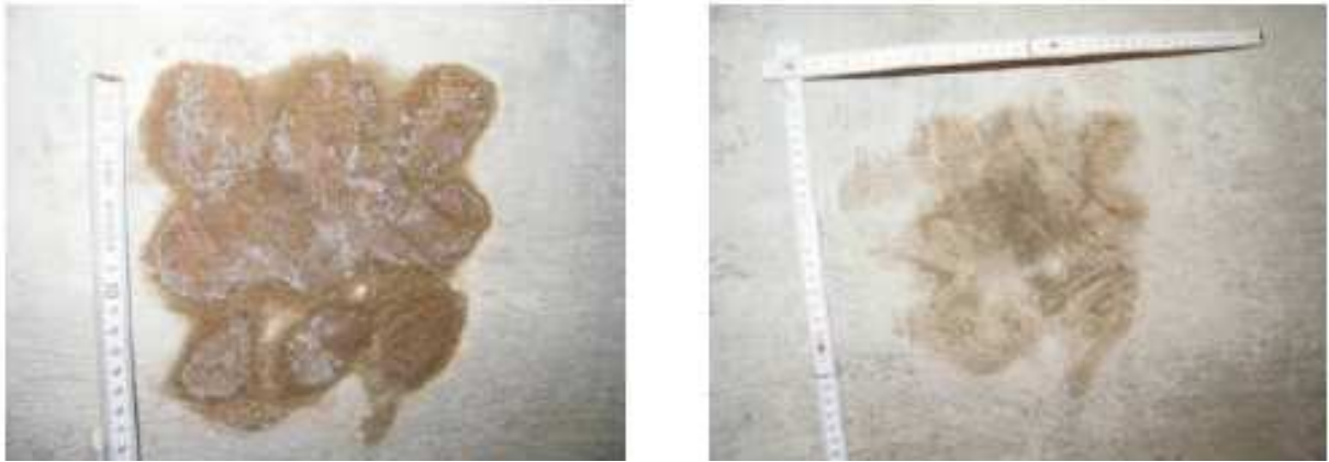
Photo 6: Change of color and expansion of the damaged area within approximately 13 weeks.
